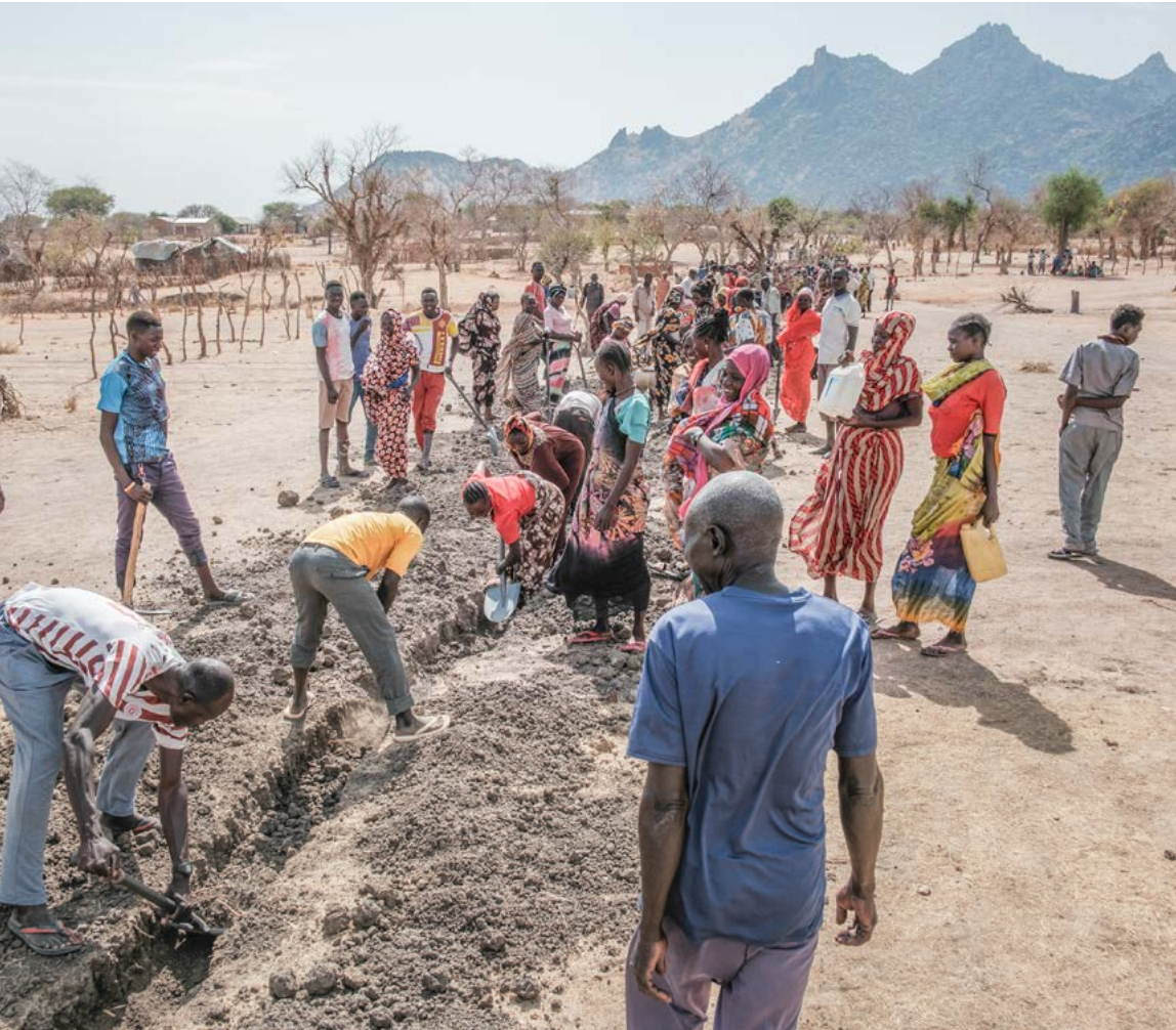
April 2025, Tungoli, Sudan. Residents of Al-Hilu IDP camp work together to dig a trench from nearby Tungoli town to the camp to lay a water pipe so people no longer need to walk all the way to the town for water where 12,000 people displaced by the war in Sudan now live in Tungoli on April 23, 2025.
